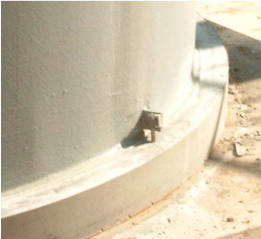
Figure 4 Readily grouted chimney base with ground connection.
