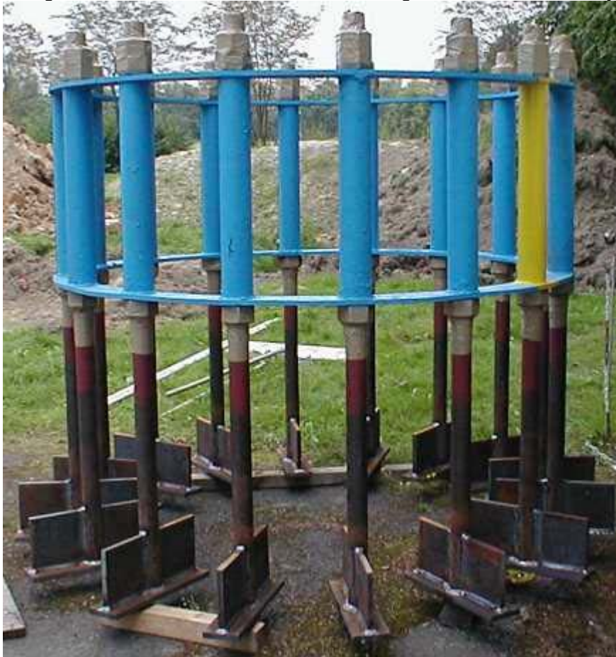
Figure 1 Anchor cage readily assembled, free thread ends and nuts covered with adhesive masking tape.
